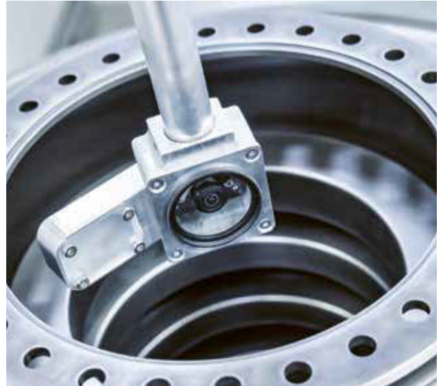
Camera track — The camera system moves inside the rotor and documents whether everything there is up to scratch and if the nuts have been tightened correctly.
